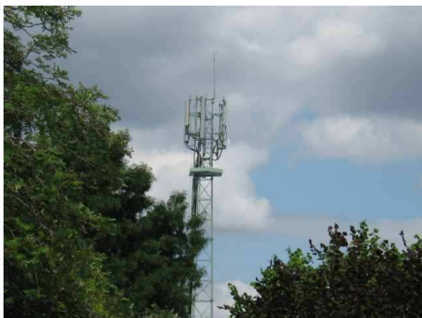
Figure 1 . Station de base 1
